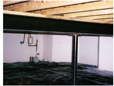
Photo 4: Conditioned crawlspace. This is the way all crawlspaces should look—dry, warm, part of the house, not part of the outside or part of the ground. Insulated on the perimeter, not in the floor. Beautiful.
