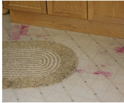
Photo 3: Vinyl flooring. Pink spots are due to moisture problems arising from the impermeability of the vinyl flooring and ventilated and insulated crawlspace underneath.
